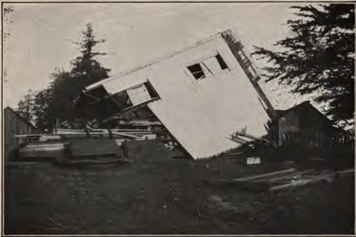
A. A TANK-HOUSE IN THE SANTA CRUZ MOUNTAINS, OVERTURNED DURING THE EARTHQUAKE OF CALIFORNIA ON APRIL 18, 1906, WITH THE FOUNDATION NOT BROKEN. (After a photograph by Fairbanks.)
